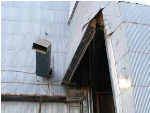
Raised truck box damages elevator door in Alvarado, MN 2009
