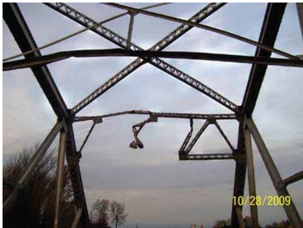
Bridge damaged by raised truck box near Thompson, ND; on the Red River, 2009
